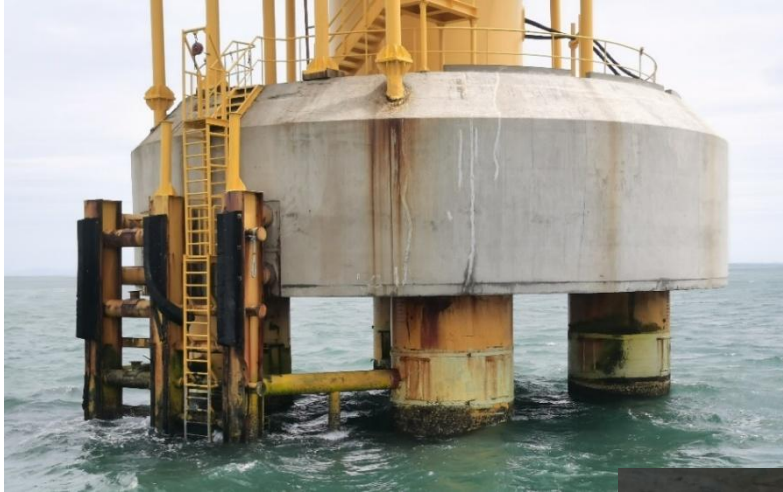
Before M&R Corroded Splash and tidal Zone
